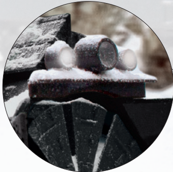
Work lights and line signal lights digitally controlled
